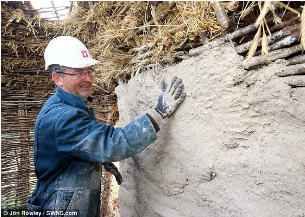
Figure 7: Example of mortar application on thatch construction frame. Source Jon Rowley SWNS.com
